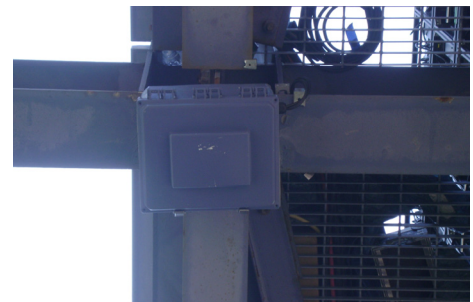
Installed Solution at the Stadium
